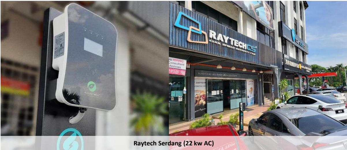
Stesen Pengecasan EV Tepi Jalan (On Street Parking)
