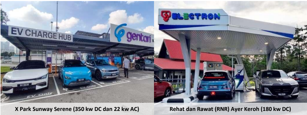
Hub Stesen Pengecasan EV
